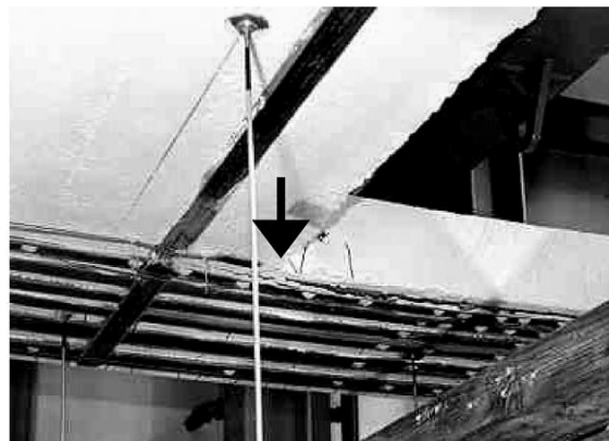
(b) Onset of strip debonding near cutout
