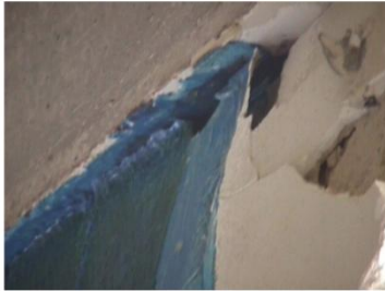
Figure 10: Delamination of Plaster in Wall 6
