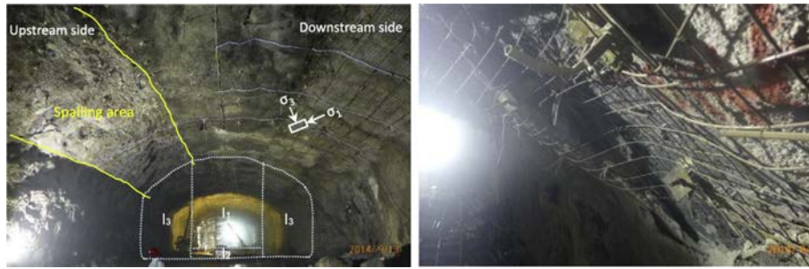
Fig. 20. Spalling in the upstream roof of the left bank powerhouse during excavation of layer I (Liu et al., 2017).
