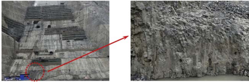
Fig. 1. Baihetan hydroelectric dam foundation (The marked area is the columnar jointed rock mass).
