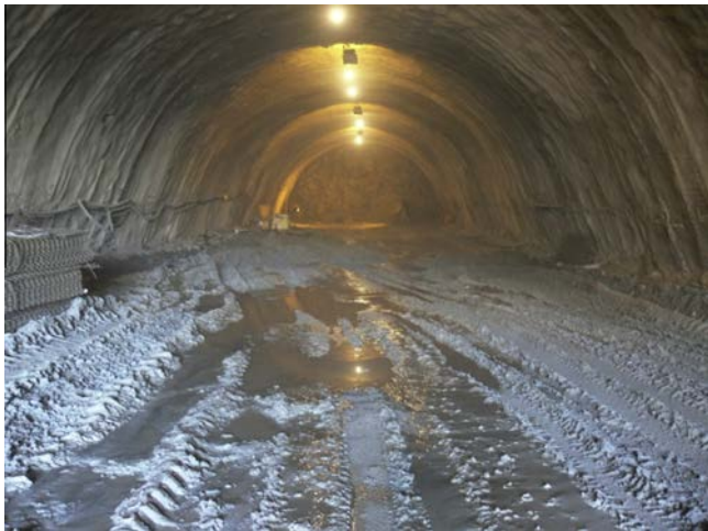
Fig. 10. The water inflow to tunnel.
