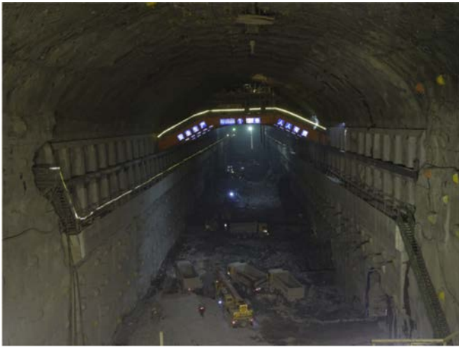
Fig. 2. Baihetan hydroelectric underground powerhouse.
