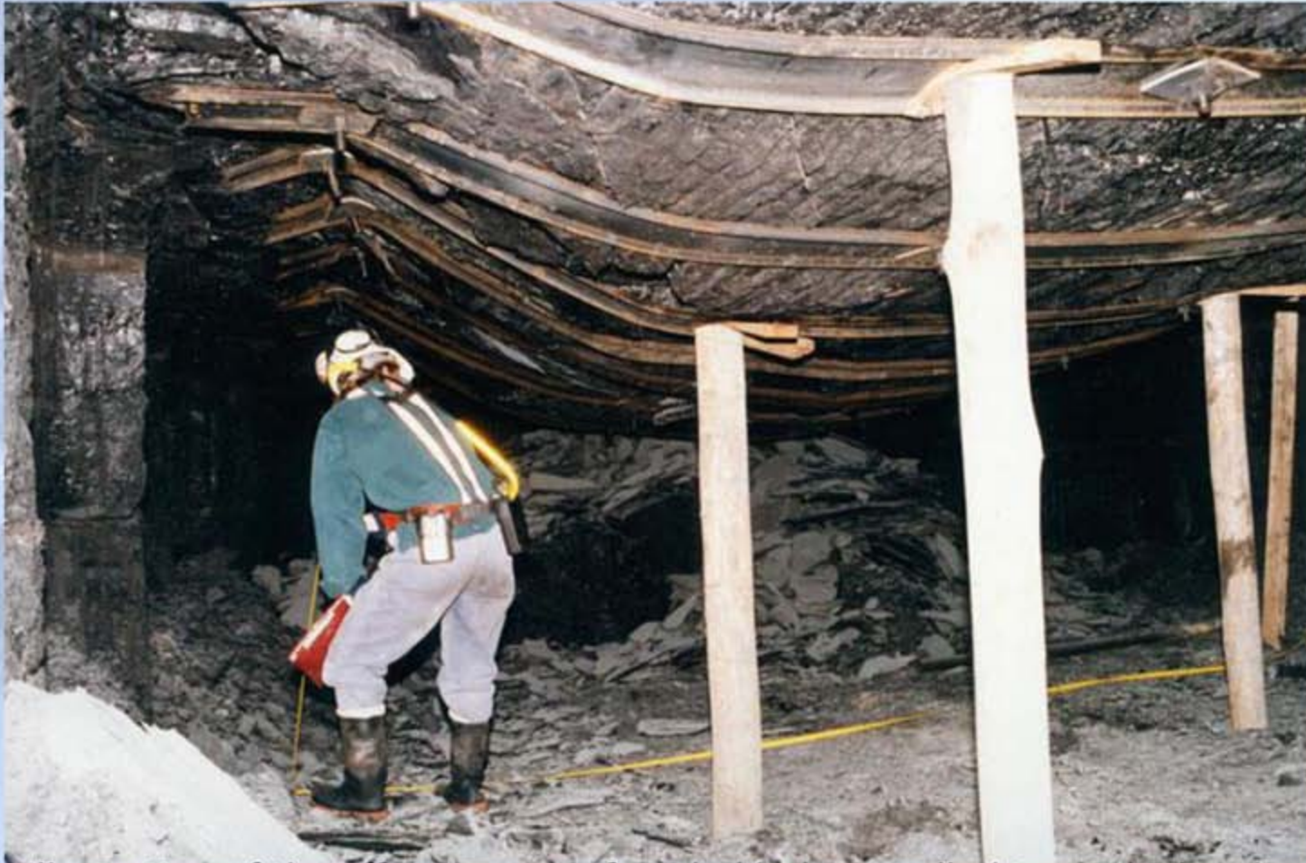
An illustration of the effectiveness of angled bolts installed towards the abutment in controlling failure of a laminated coal roof
