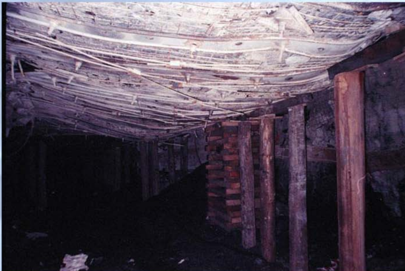
An example of failed immediate roof suspended off the excavation abutments by means of long tendons angled over the ribline and trussed across the excavation
