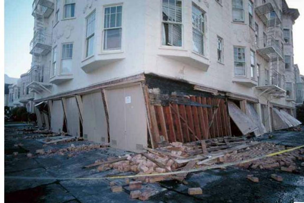
Loma Prieta earthquake damage in San Francisco. The soft first story is due to construction of garages in the first story and resultant reduction in shear strength. (Photo from: http://earthquake.usgs.gov/bytopic/photos.html )
