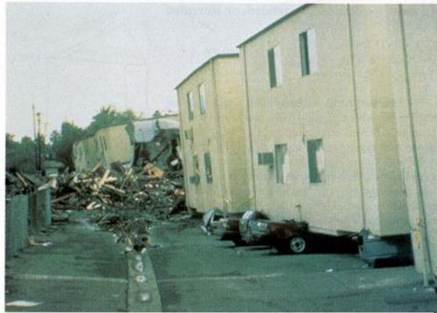
Northridge earthquake soft first story (parking level) damage. (Photo from: Brown, R.D., Jr., Lessons reaffirmed, extended, or revealed, Earthquakes and Volcanoes , Vol. 25, No. 2, 103-106, 1994)
