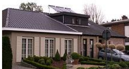
A solar water heater installed on a house in Belgium
