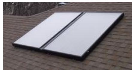
Flat-plate solar thermal collector, viewed from roof-level
